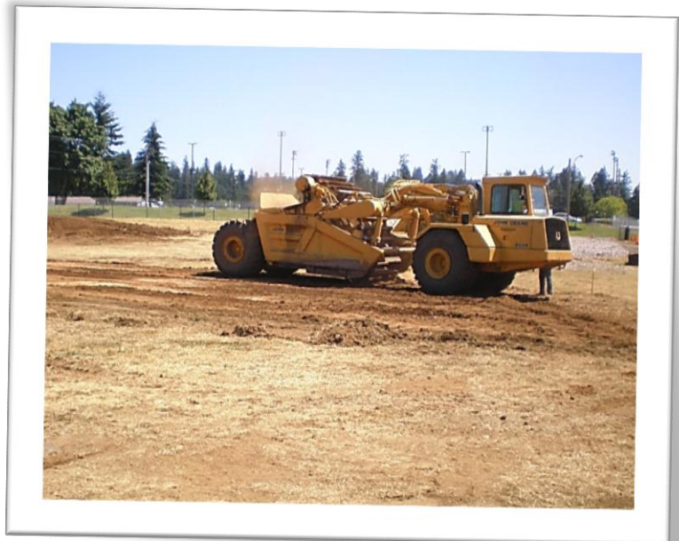
Columbia West overseeing grading and compaction activities at Helen Baller Elementary School.
